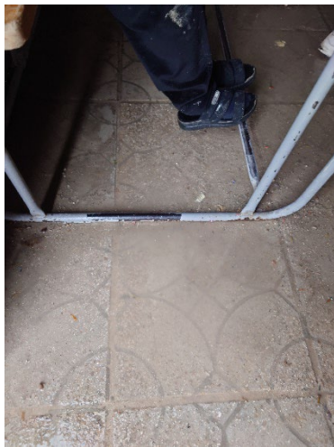
Photo 6 Water leak on a rainy day
